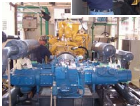
Trillium has installed new Ariel compressors at the Jackie Gleason depot in Brooklyn, N.Y.
